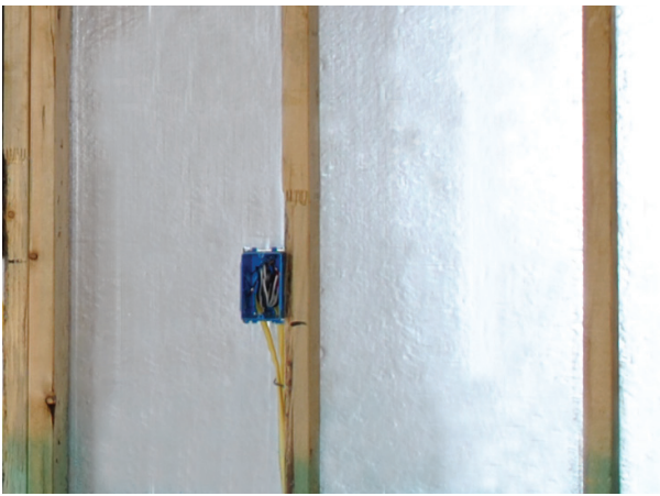
External wall with sealed joints where electrical boxes are inside the air barrier.
