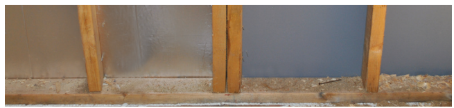
Corners and joints are sealed with external tape. Only top and bottom plates require additional sealant.
